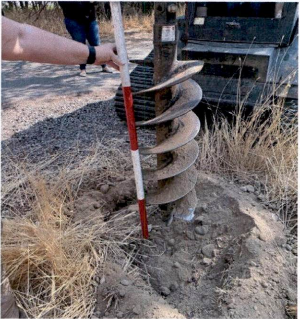
Figure 10. Soils were uniformly loose sand and cobbles, too unstable to allow for a "clean" excavation.
